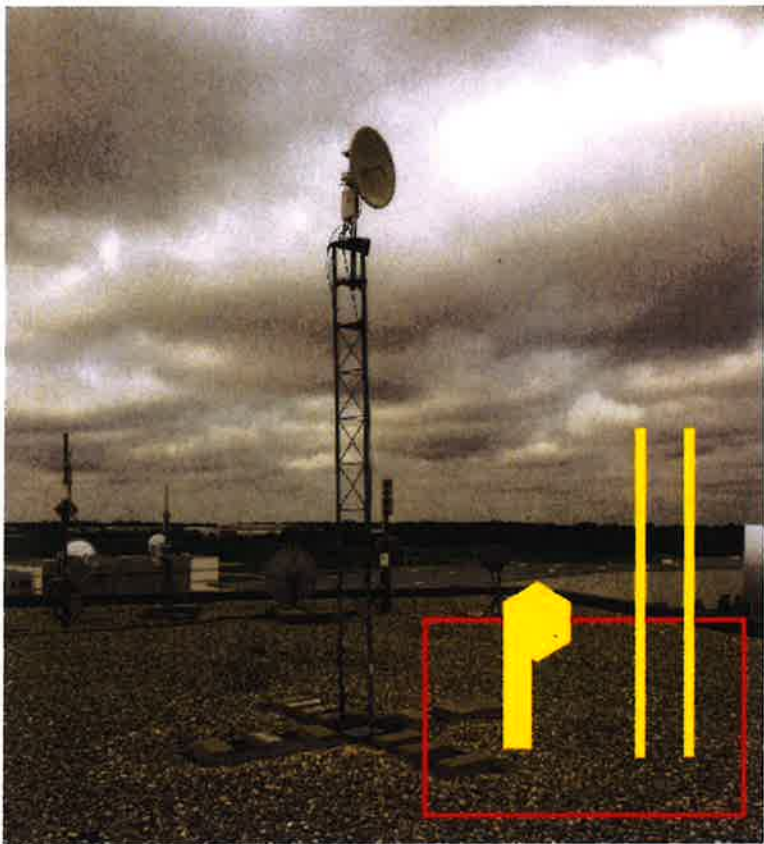
Reserved Space for Future Public Safety Communication Equipment Flight Center Roof 2700 International Drive – West Chicago, IL
