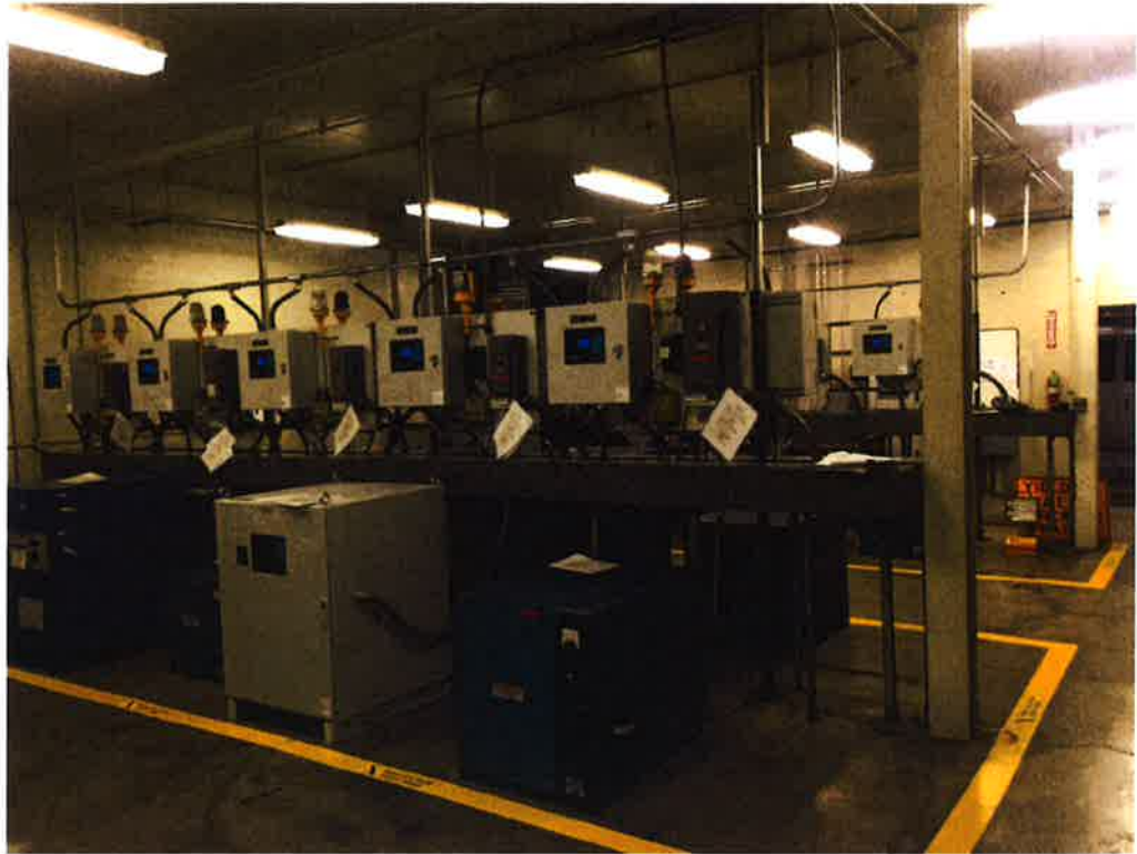
Airfield Electrical Vault – DuPage Airport Maintenance Building
