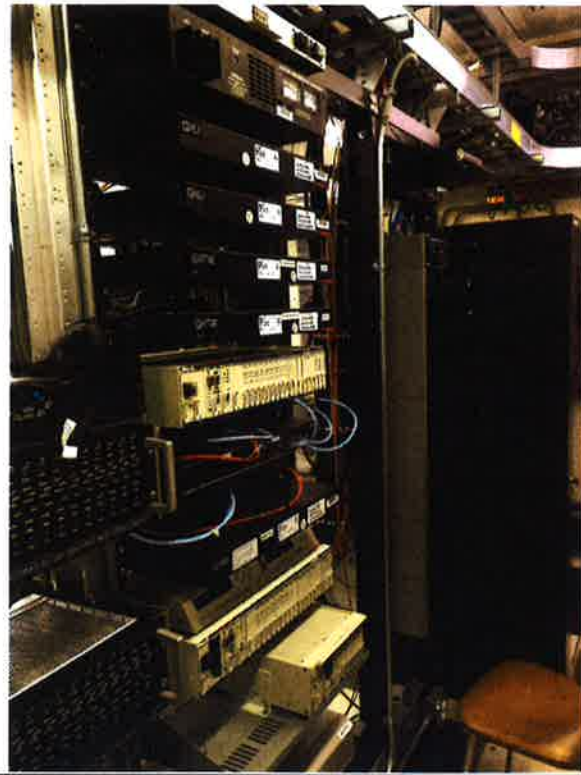
Building 170B Communications Equipment Room 170 Wall Street – Glendale Heights, IL
