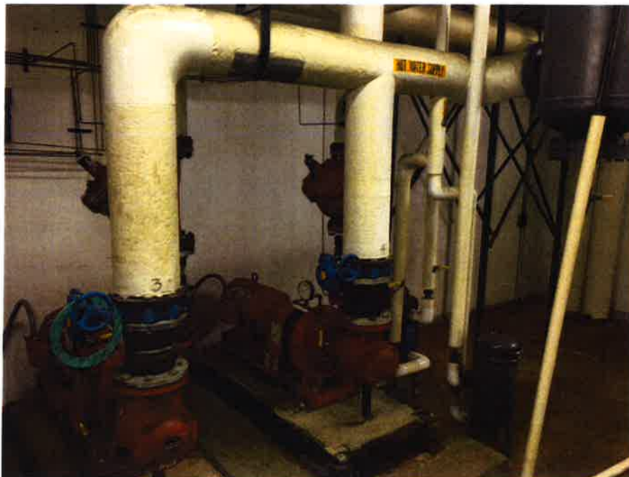
Existing Hot Water Pumps
