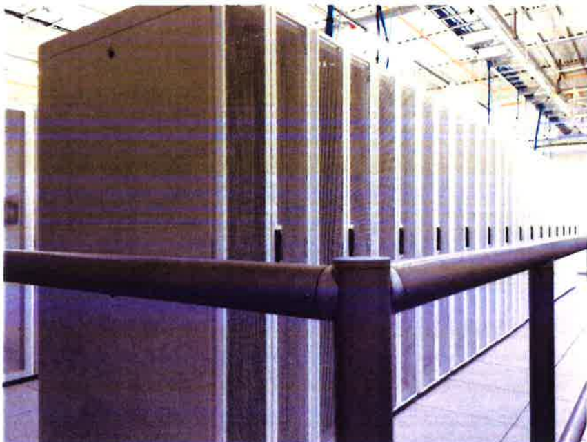
Netrix Data Center (Off-Site Backup) – Mt. Prospect, IL
