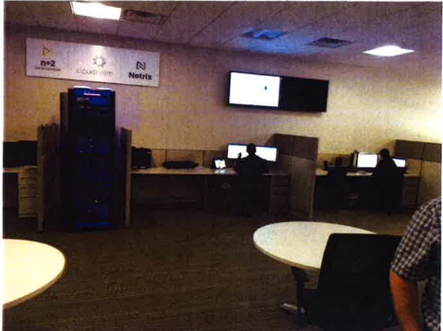
Netrix 24/7 Network Operations Center Monitoring Station – Mt. Prospect, IL
